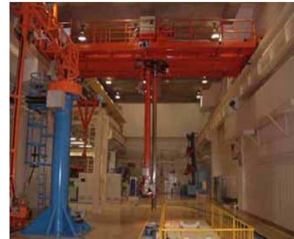
Remotely controlled assembly transferring and assembly storage
